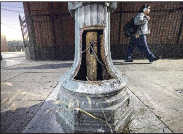
ON BROADWAY and 23rd in downtown, cut wires can be seen from one of L.A.’s historic streetlights.
